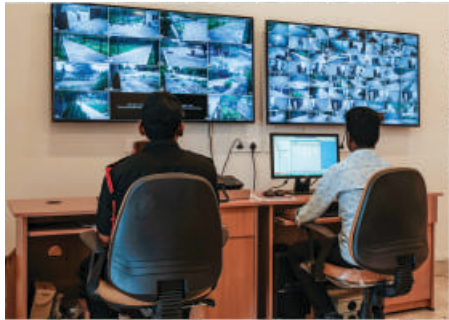
CCTV Control Room
